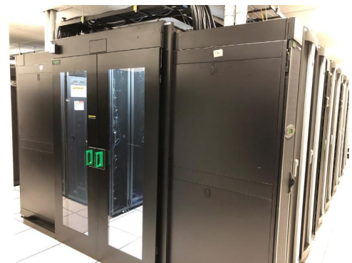
[Before and after implementation of pod hot-aisle containment system.]
